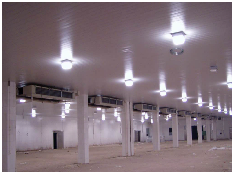
Figure 15: Large-scale refrigerated warehouse
